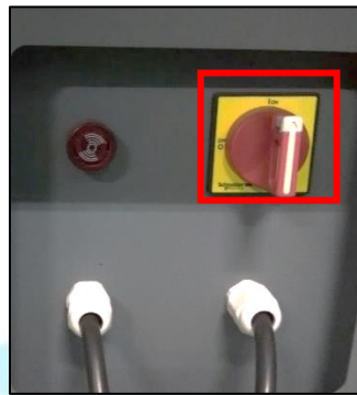
Figure 8: Turning ON the Main Power Switch
